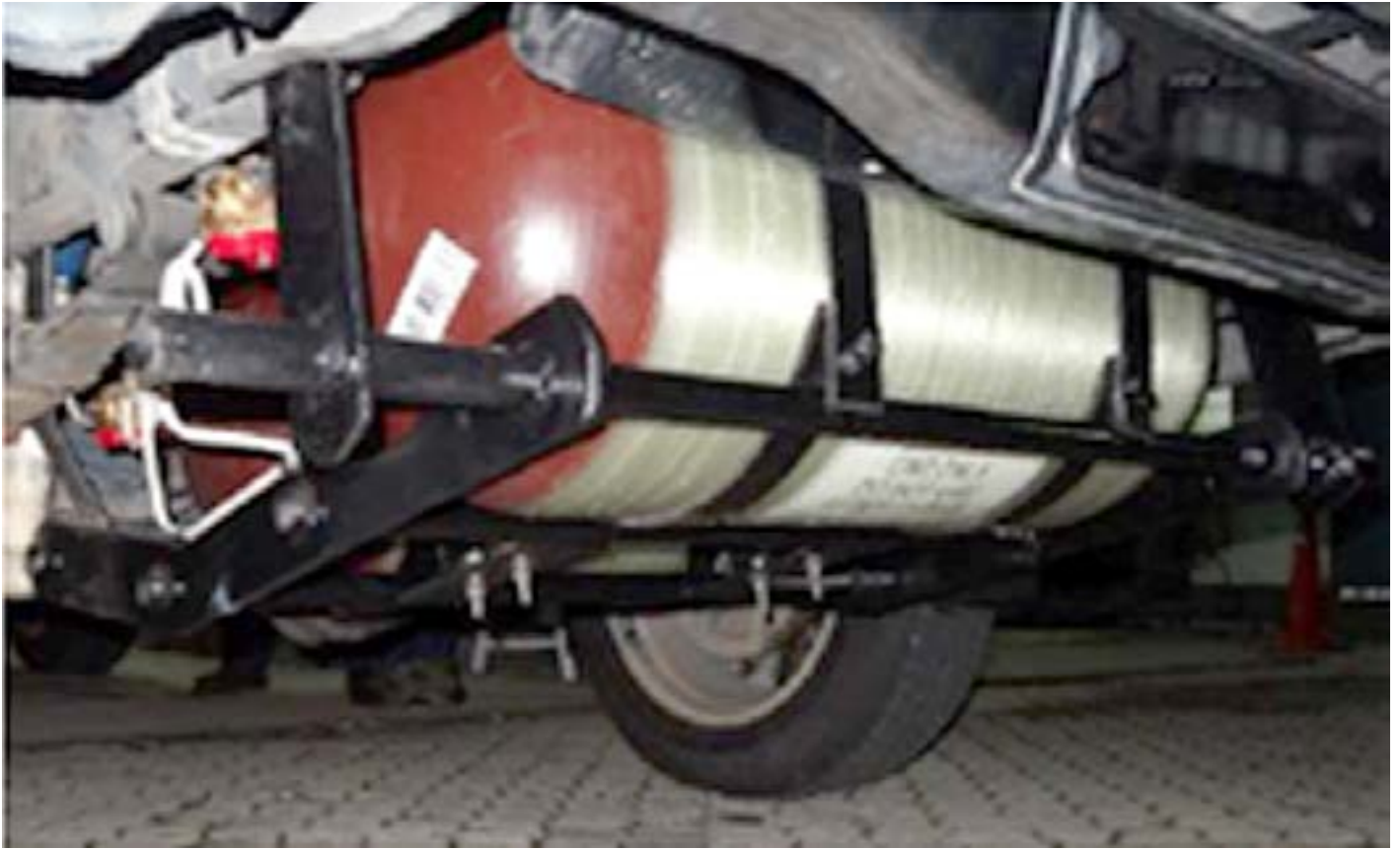
Fig. 1: CNG cylinder installed
